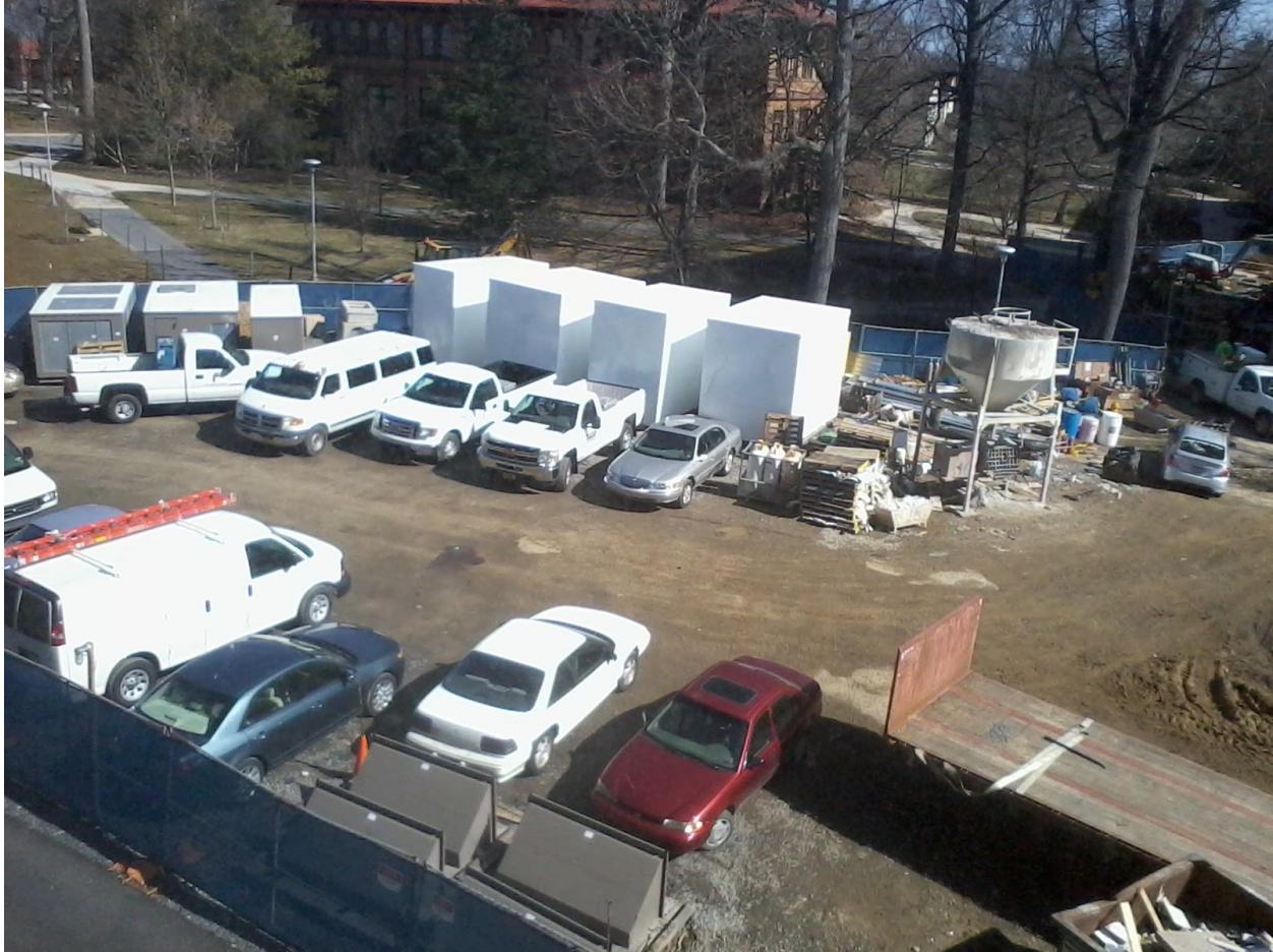
Figure 11: Stored mechanical equipment displacing contractor parking.
