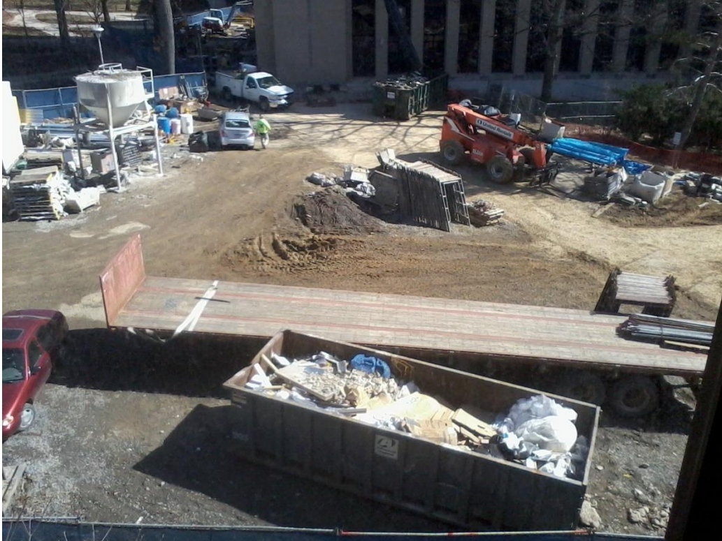
Figure 12: Stack of scaffolding and mortar mixer forced to center of site. Semi-trailer blocks the dumpster.
